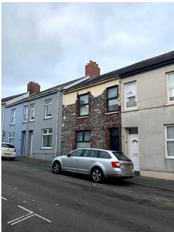
A terraced house on Parcmaen Street with its render partially removed, revealing the grey rubble stone and red brick window and door surrounds beneath.
