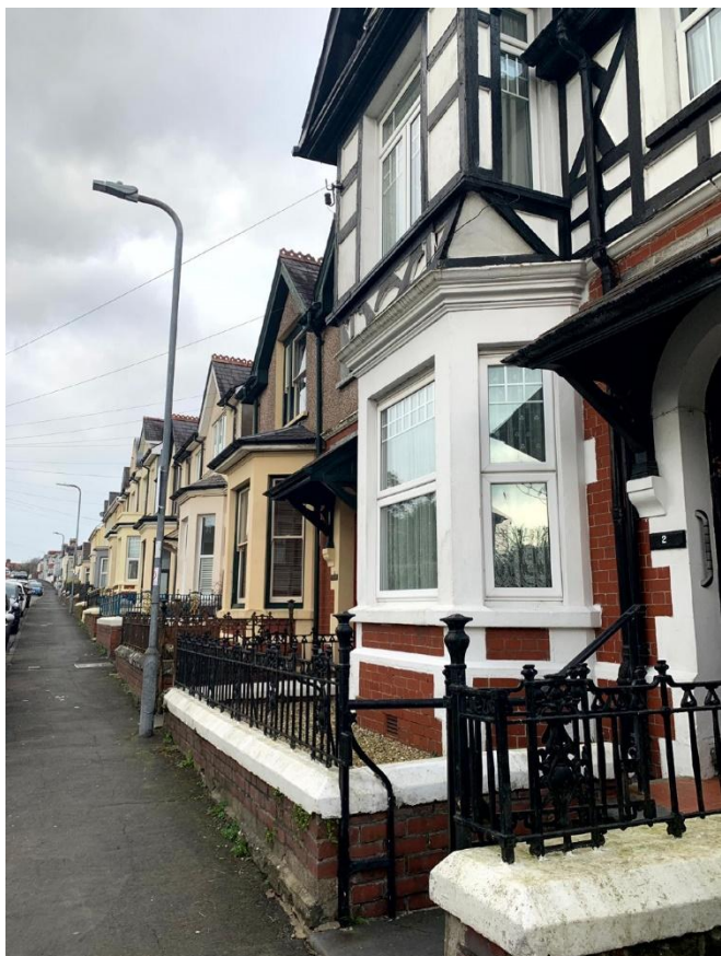
The wrought iron railings to the semi-detached houses on the St David's Avenue
