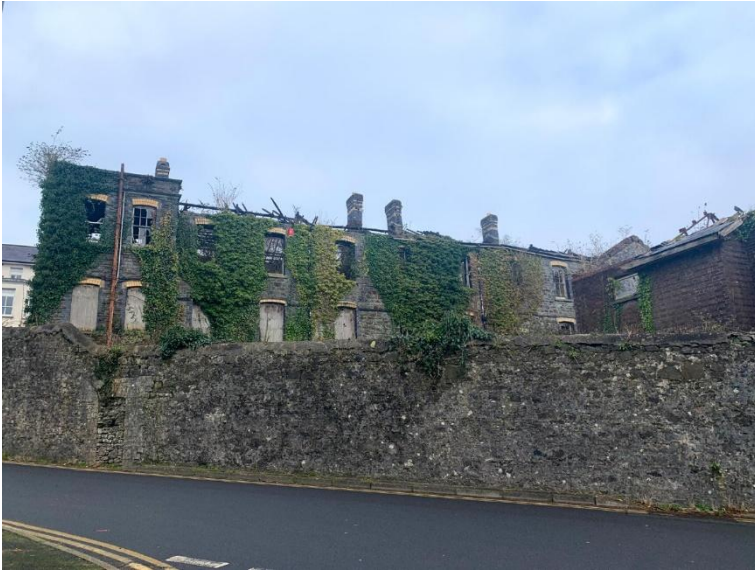
The southern building of the historic workhouse site in a ruinous condition.
